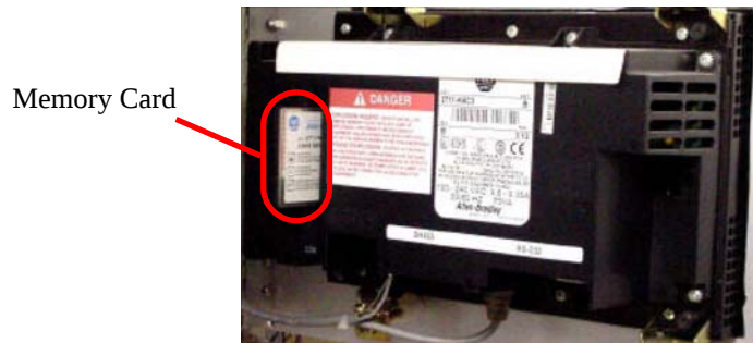
Figure 18. Operator Terminal (Rear)
